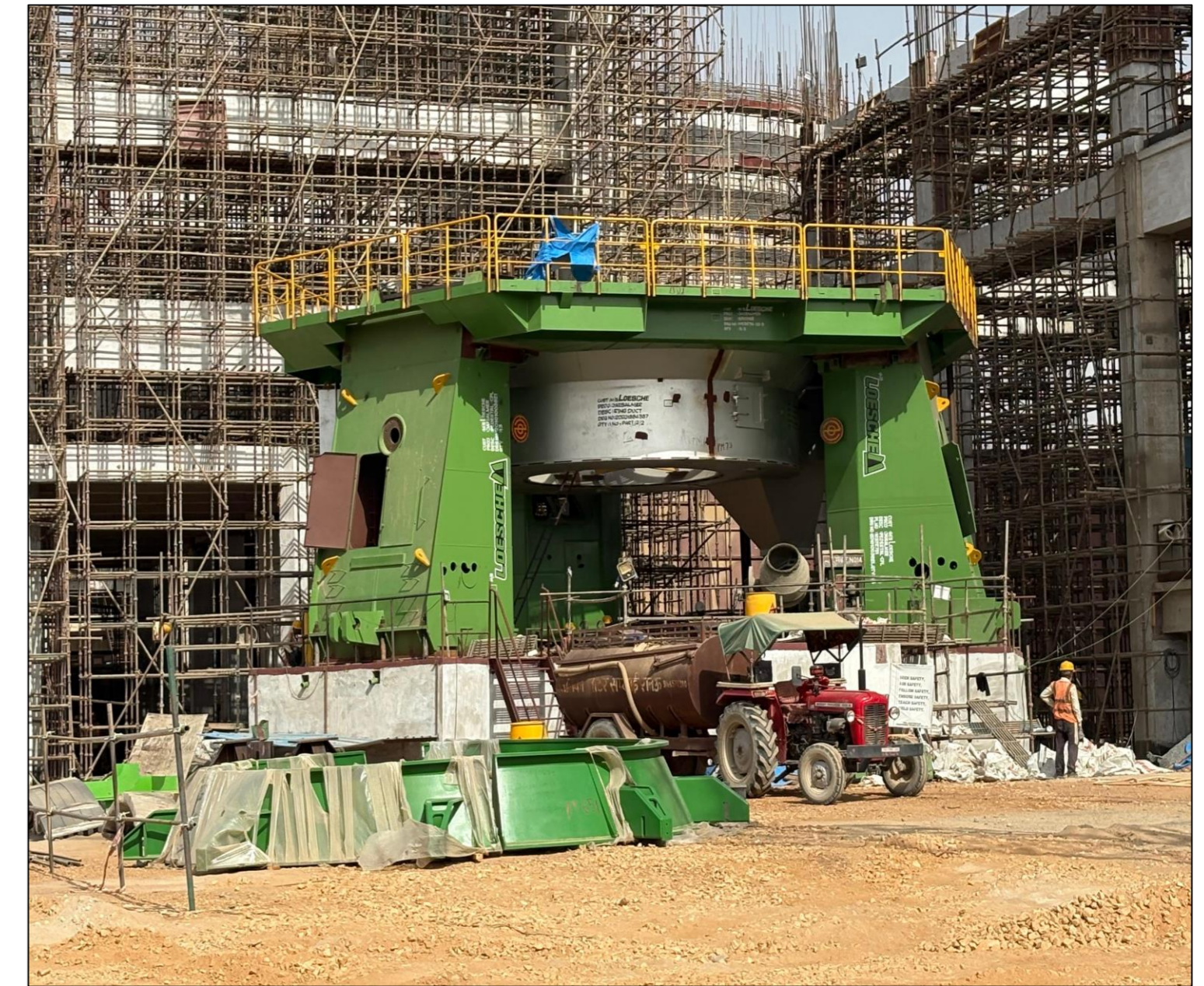
Cement Mill VRM
