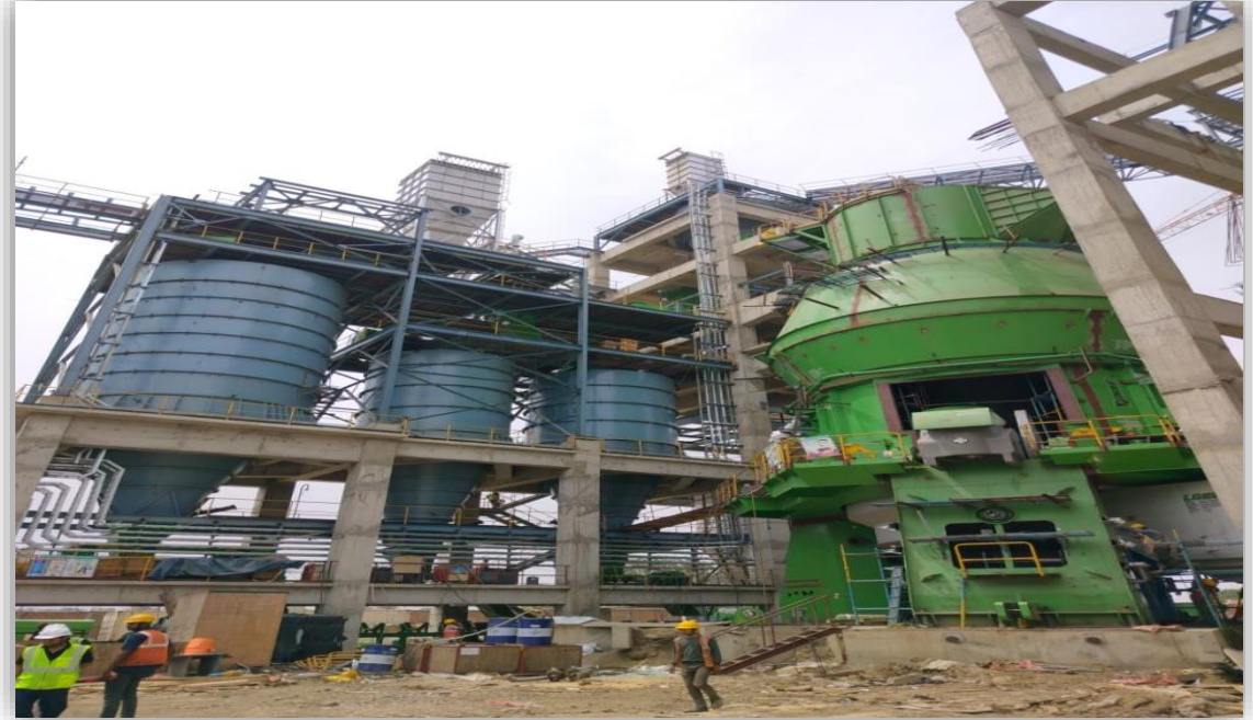
Hopper & Cement Mill
