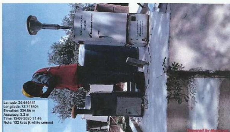
132 KV Sub Station
