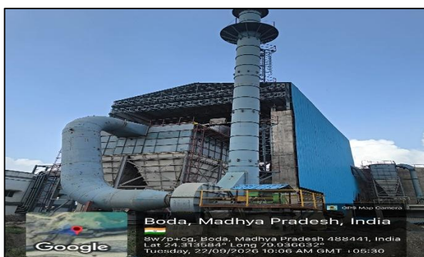
Crusher equipped with Bagfilter
