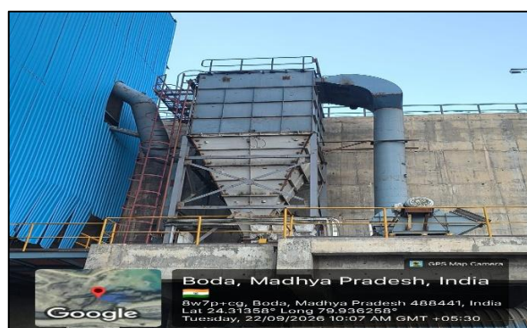
Bag filter installed at transfer point
