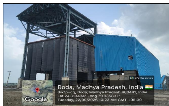
Belt Curtain at crusher hopper
