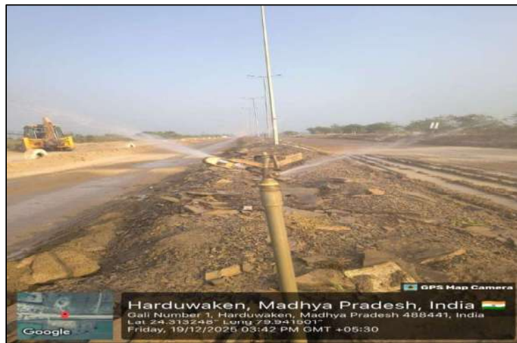
Permanent water sprinkler at haulage road
