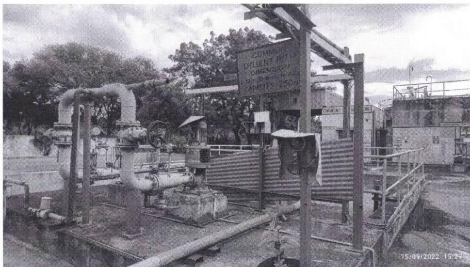
ETP installed at CPP
