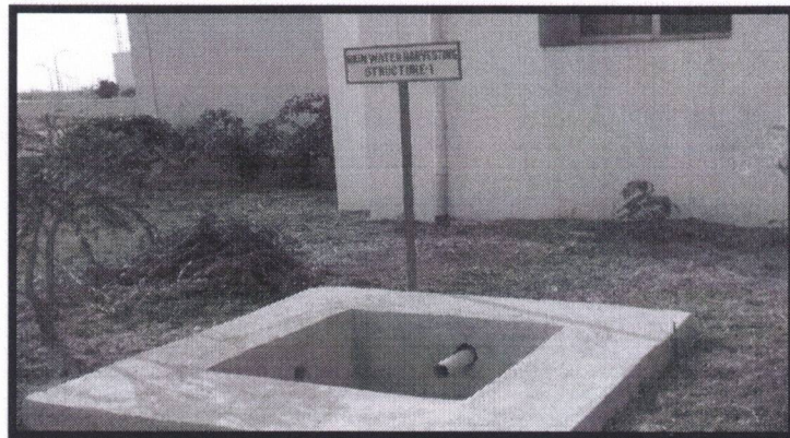
Rainwater Recharge Pit
