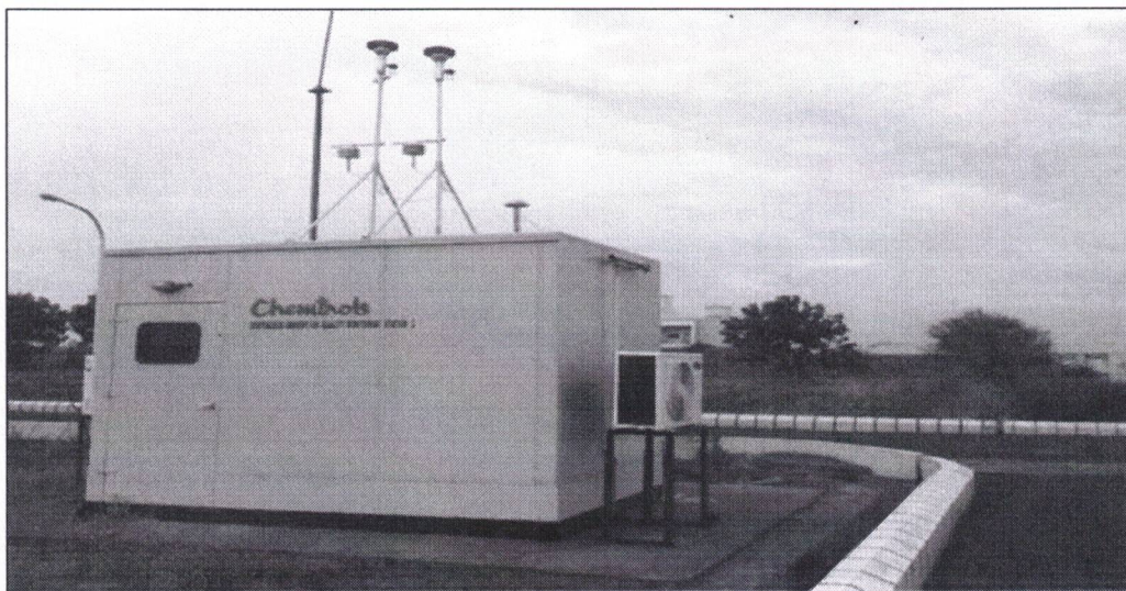
CAAQMS installed at Colony
