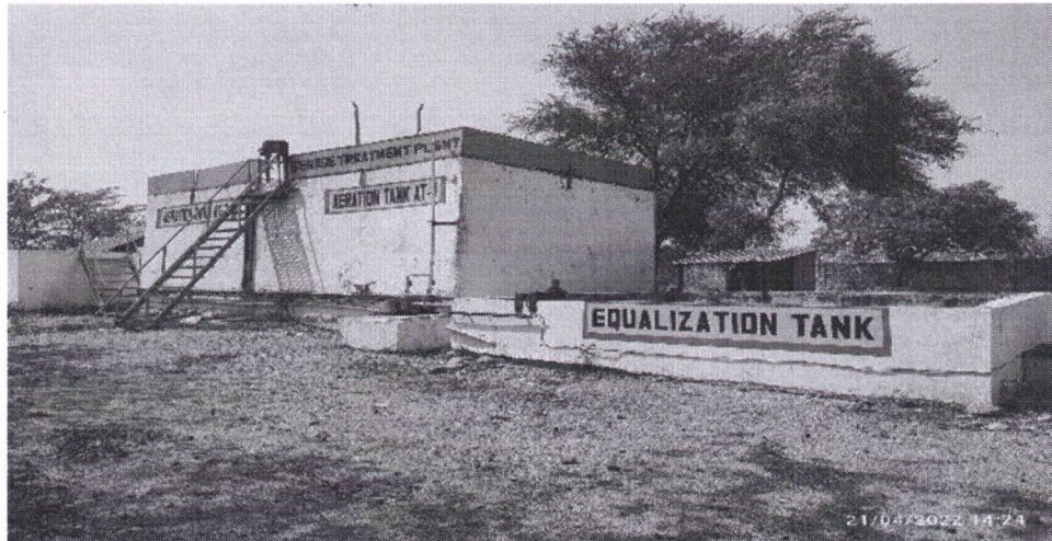
STP installed at Plant
