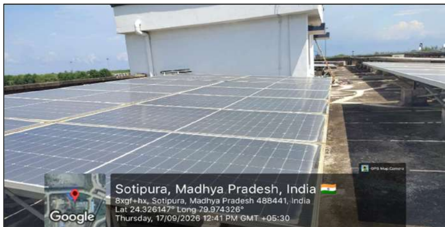
Picture 5- Roof top solar system
