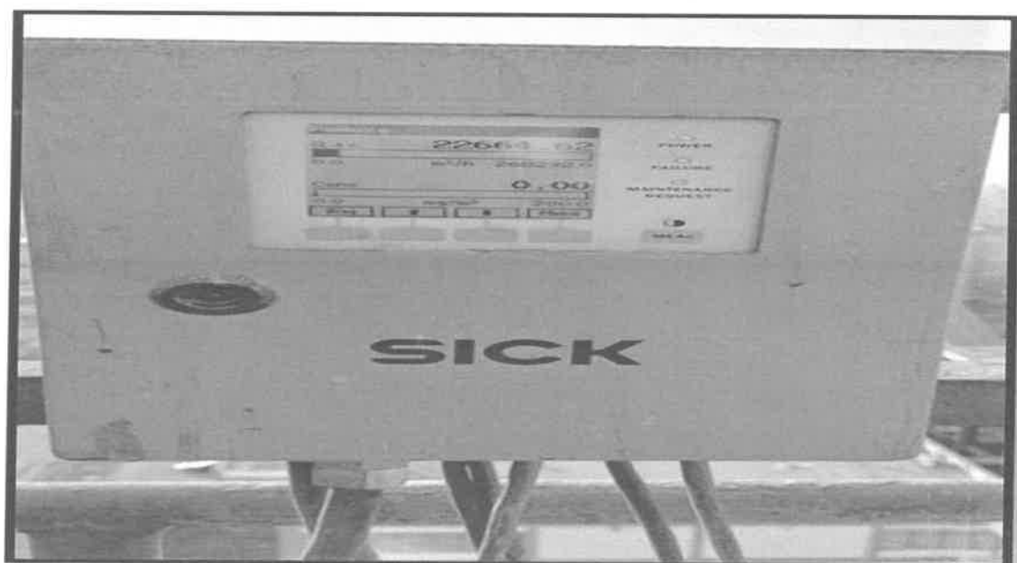
Picture 7- Continuous Emission Monitoring Systems (CEMS) installed
