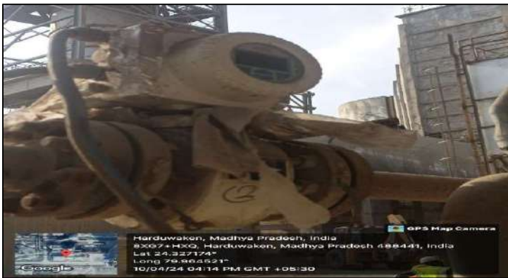
Cooler spray meter
