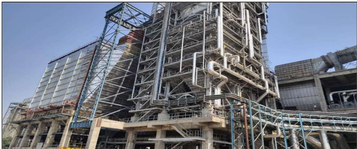
Waste heat recovery system
