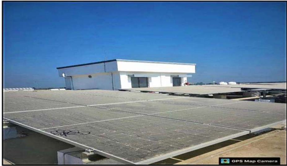
Solar power generation on admin building of roof top:
