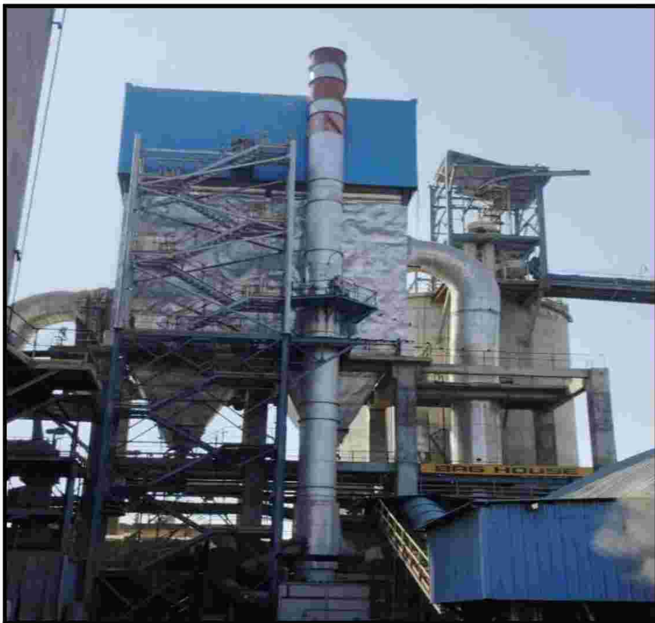
Bag house is fully insulated
