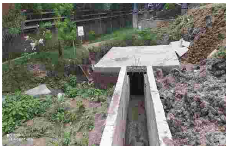
Rain water recharge pit No.-03
