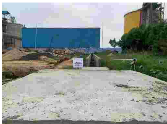
Rain water recharge pit No.-04
