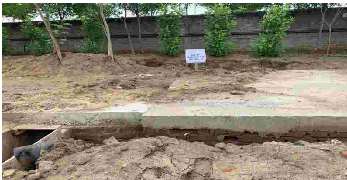
Rain water recharge pit No.-05
