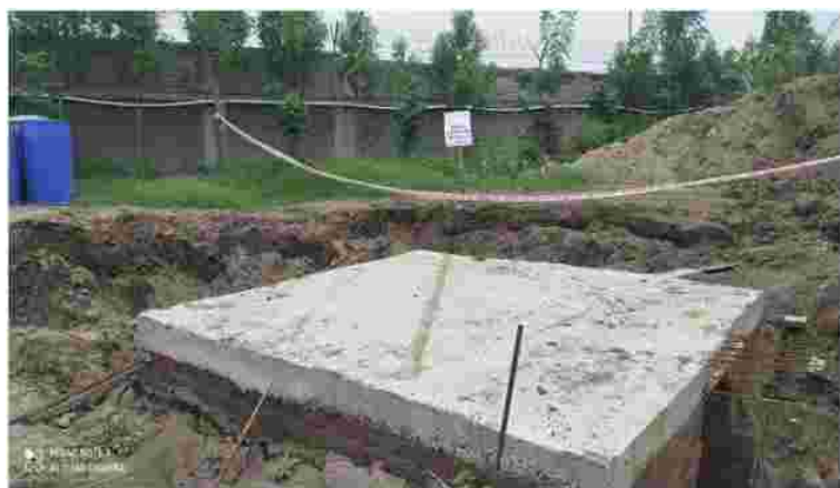
Rain water recharge pit No.-01
