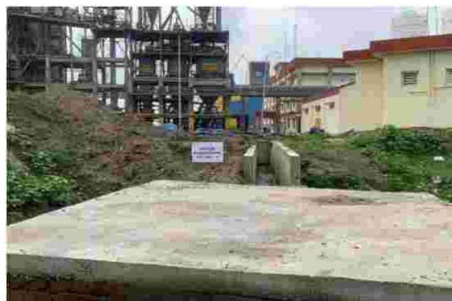
Rain water recharge pit No.-02
