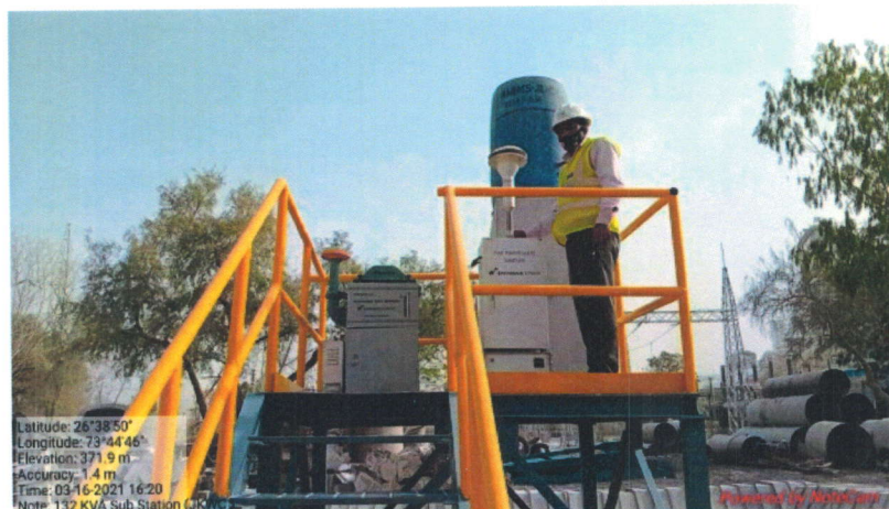
132 KV Sub Station
